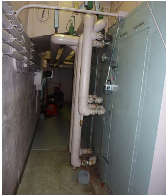
Air Handler #1 And Piping To Heating And Cooling Coils
