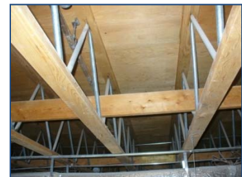
Photo no. 4 – TjL joists framing in the 2 nd floor of Actors Wing.
