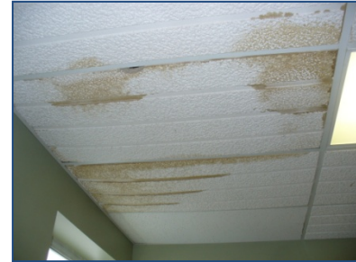
Photo no. 7 – Water stain in ceiling tiles indicating possible leaks from above. Further investigation is required to determine cause.
