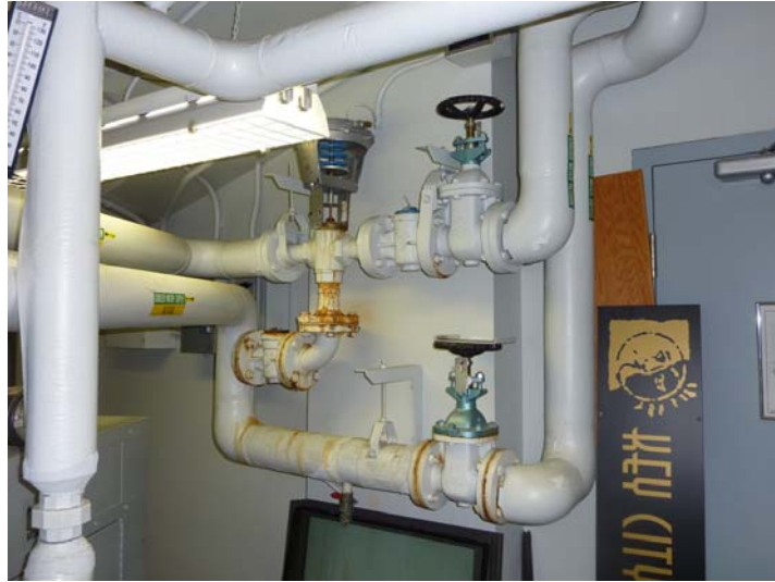
Chilled Water Piping – Air Handling Unit #2
