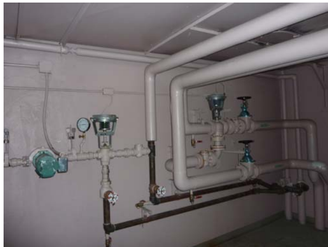
Heating And Chilled Water Piping Air Handling Unit #1
