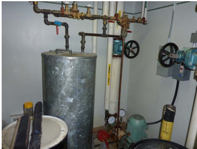
Glycol Tank, Chilled Water Pump and Piping for Chilled Water System
