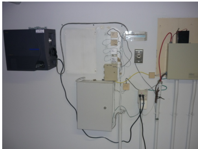
Telephone and Security
