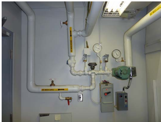
Heating Piping Air Handling Unit #2
