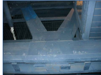
Photo no. 11 – Timber truss not strengthened.
