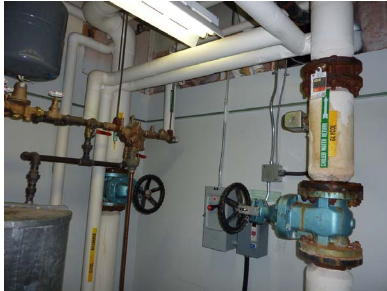
Chilled Water Piping, Valving and Components
