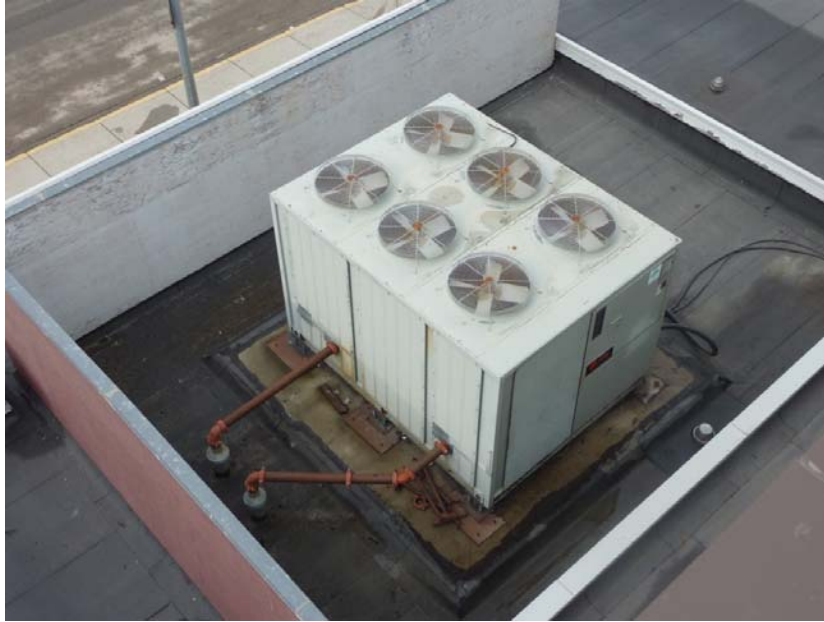
Roof Mounted Air Cooled Chiller
