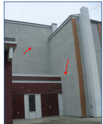
Photo no. 5 – Cracking & general deterioration of stucco in the west wall.
