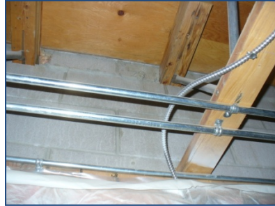
Photo no. 6 – Block wall section in joist space was un-insulated & in direct contact with the wood joists, which shows signs of water stain possibly from condensation.
