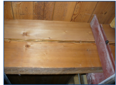
Photo no. 12 – Significant checking & warping of the secondary timber beams. Bolted connection of steel angle hangers through the crack
